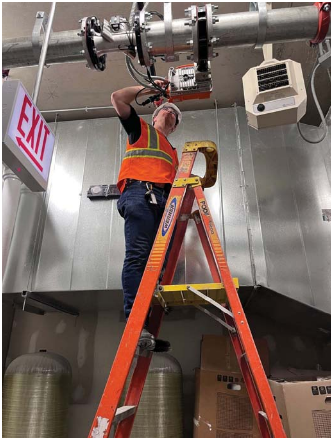
Plumbing engineers are charged with the responsibility to foresee and design water systems that are visible and operating within parameters for the lifespan of the building. Photo credit: WINT
